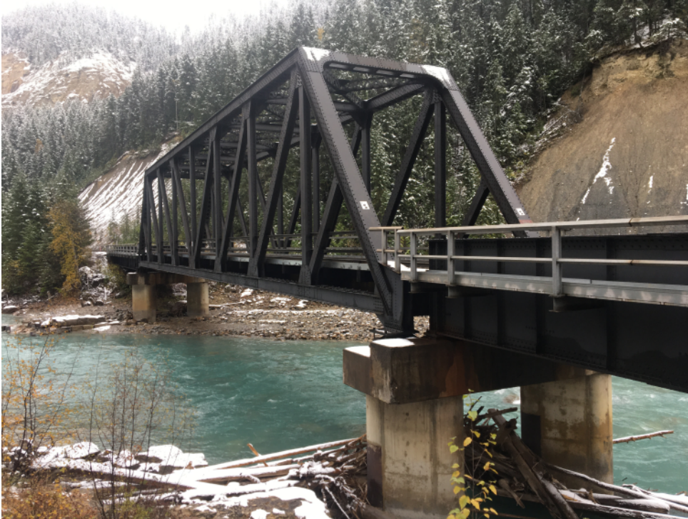
LEFT: Bridge crossing the Kicking Horse River at Mile 31.8. Photo by Rob England
